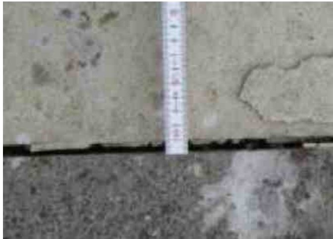
offene Fugen Bordsteine
